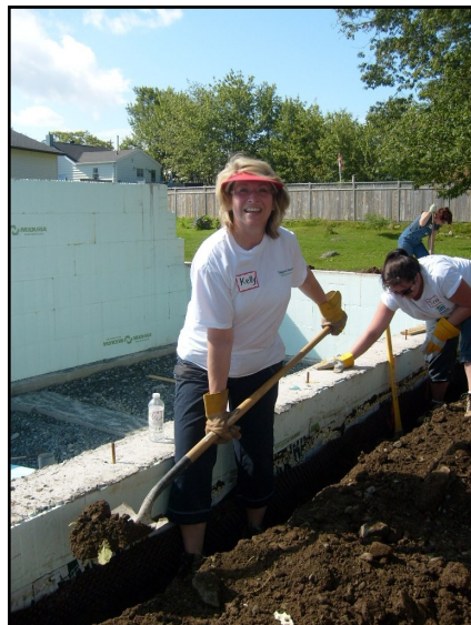
August 27, 2011 - Kelly at the launch of Habitat for Humanity's 2011 build in Spryfield. Partner families, volunteers and sponsors broke ground on a project that is building two sets of semidetached
